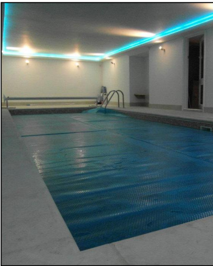
Air source heat pumps provide heating and hot water to the house and indoor swimming pool.
